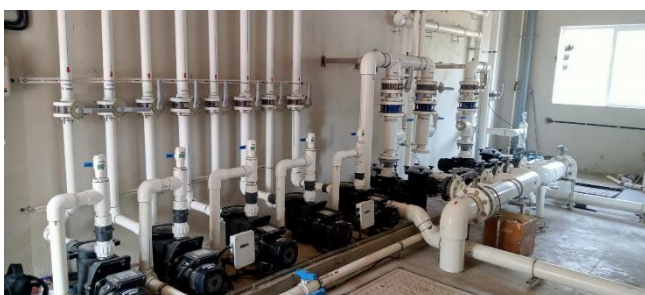
Fig.2. Equipment are placed in a well-planned manner.
