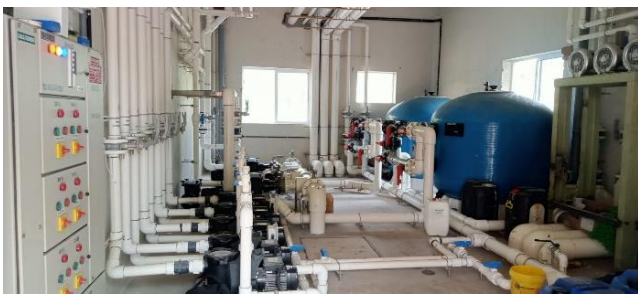
Fig.1. All equipment / pipe, supported and intactness ensured.
